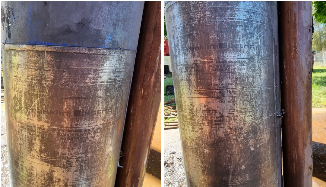
Identification plates as noted on submersible pump.
